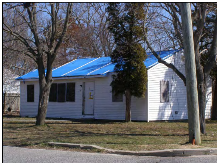
Picture 24: Boarded house
